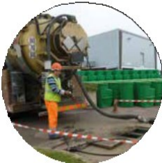
Secure the space around the opening at the time of emptying
