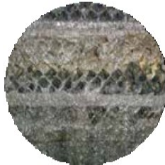
Check the components inside the oil separator and clean them if necessary
